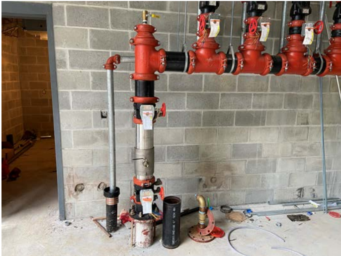
Fire protection connected to water main
