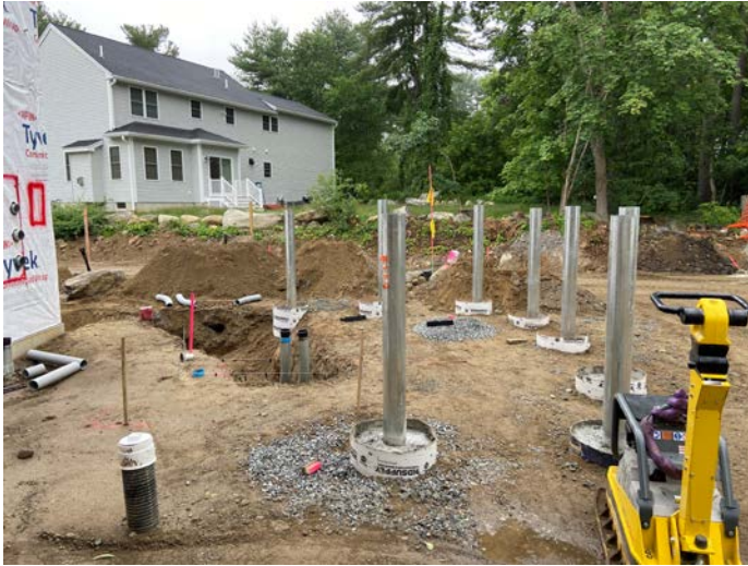
Transformer pad bollards
