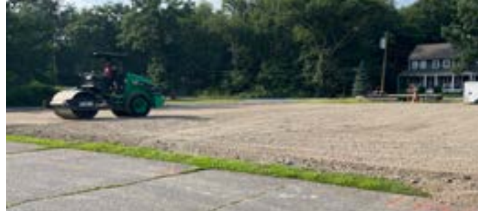
Elm Street court surface reclaimed and its new gravel base being graded
